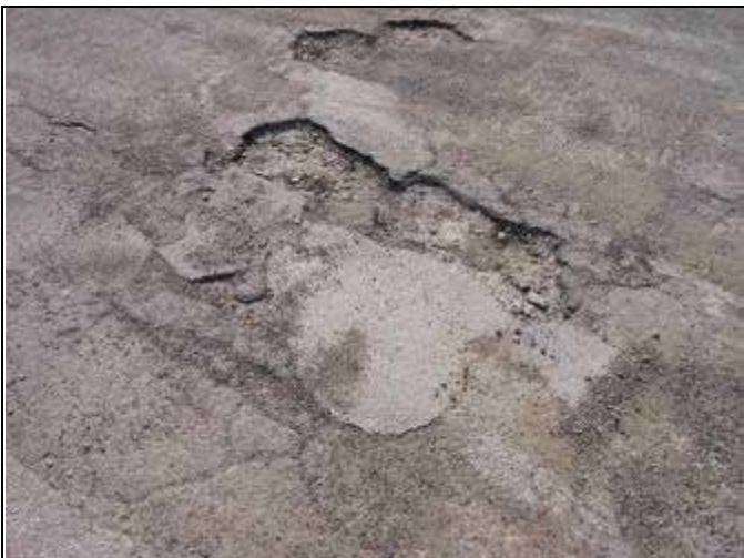
59. Pavement damage at George Haddaway Drive
