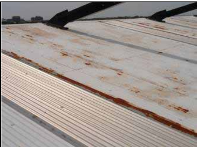
65. Roofing panel corrosion
