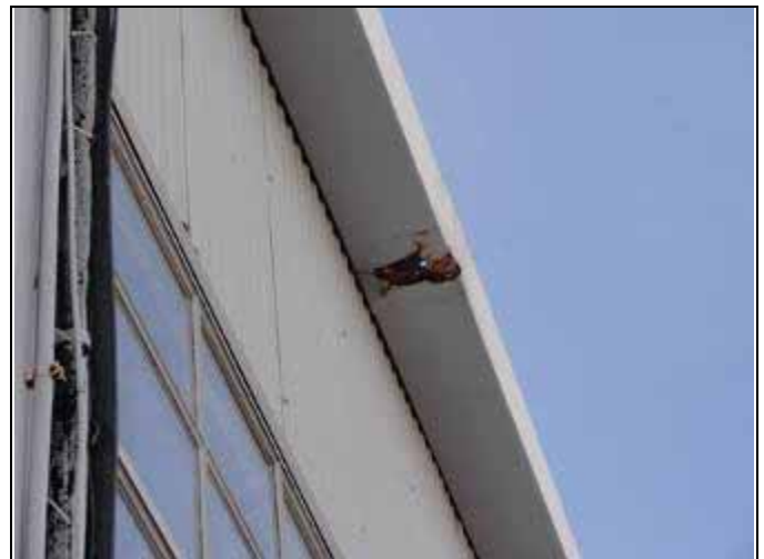
72. Corroded roof gutter
