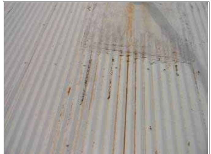
66. Roofing panel corrosion and deteriorated finish
