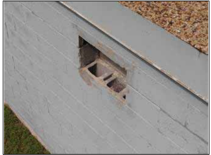
80. Damaged CMU wall at addition
