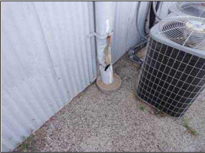
73. Damaged roof downspout
