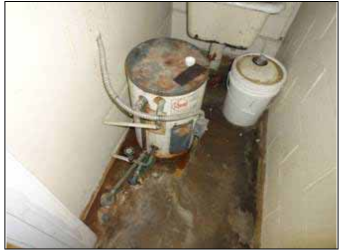
44. Domestic water heater
