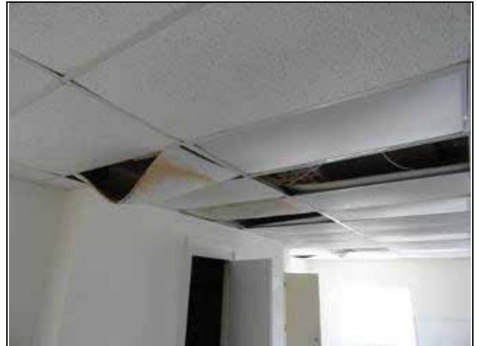
84. Damaged interior finishes
