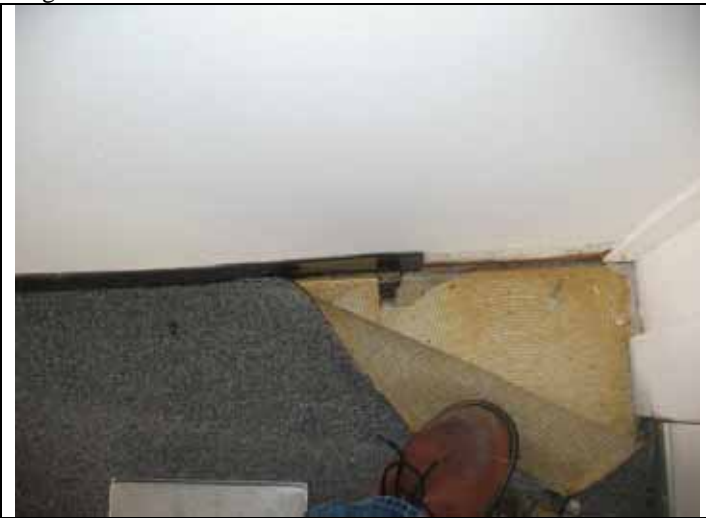
9. View of ACBM tile under non-ACBM tile, under carpet on 2 nd floor of NE office area of east hanger.
