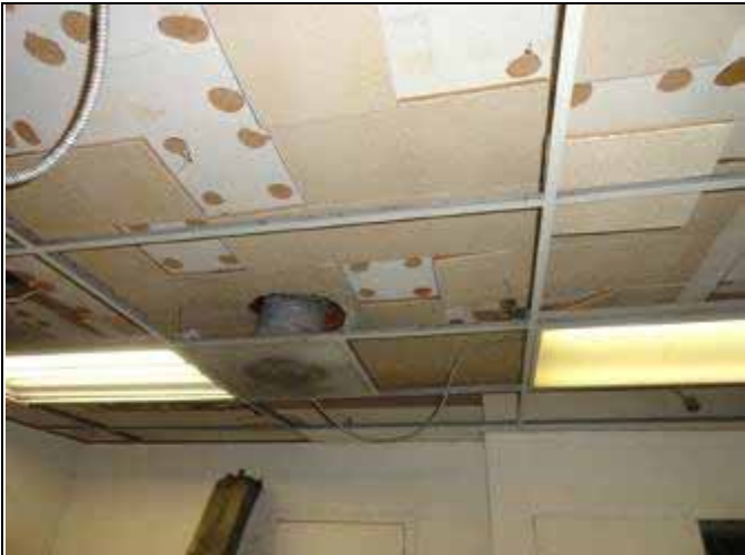
83. Damaged interior finishes
