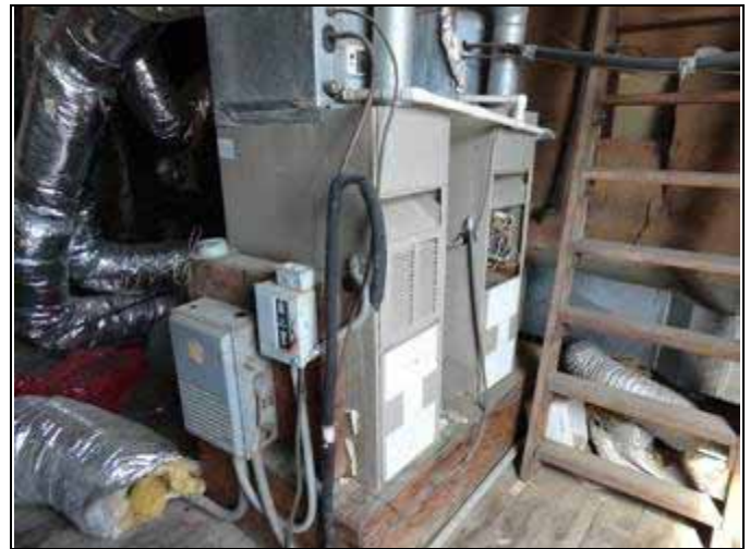
40. HVAC split system furnace
