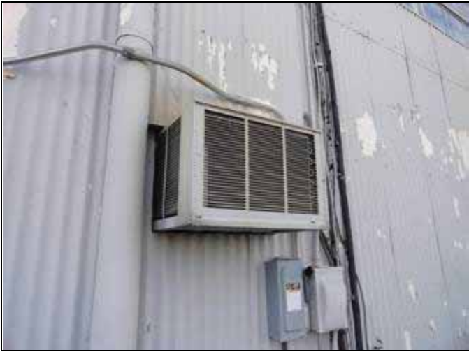
43. HVAC packaged through-wall unit
