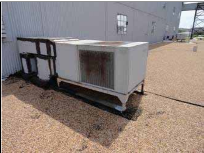
41. HVAC package unit
