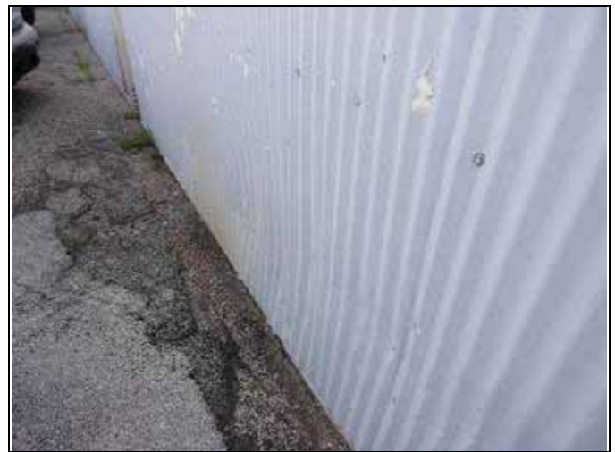
76. Impact damaged wall panels
