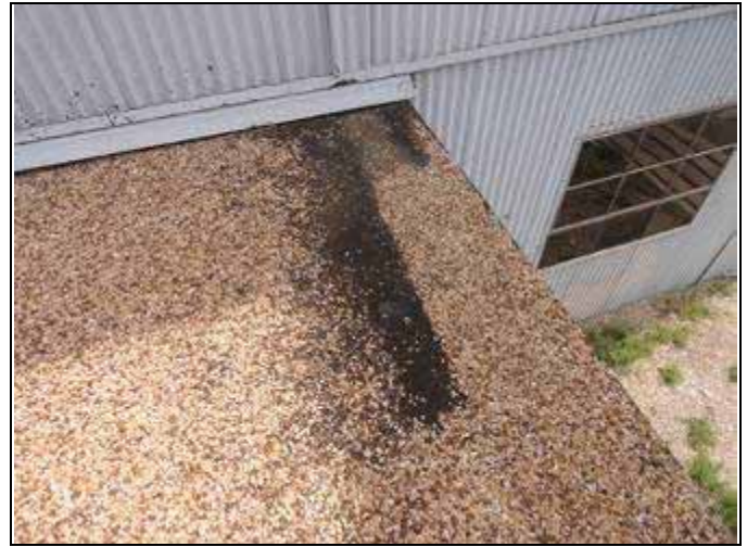
74. Displaced built-up aggregate and cracking bitumen
