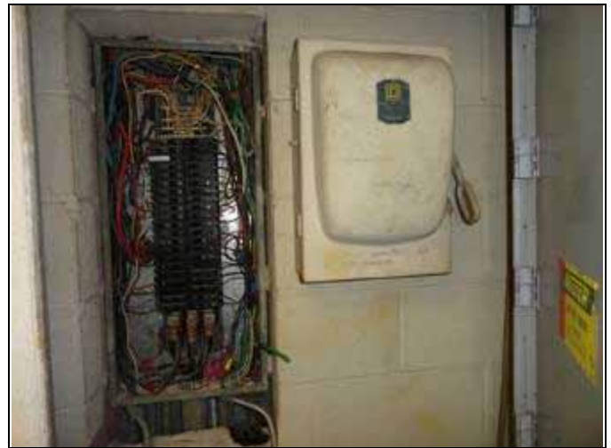
82. Exposed electrical panel wiring
