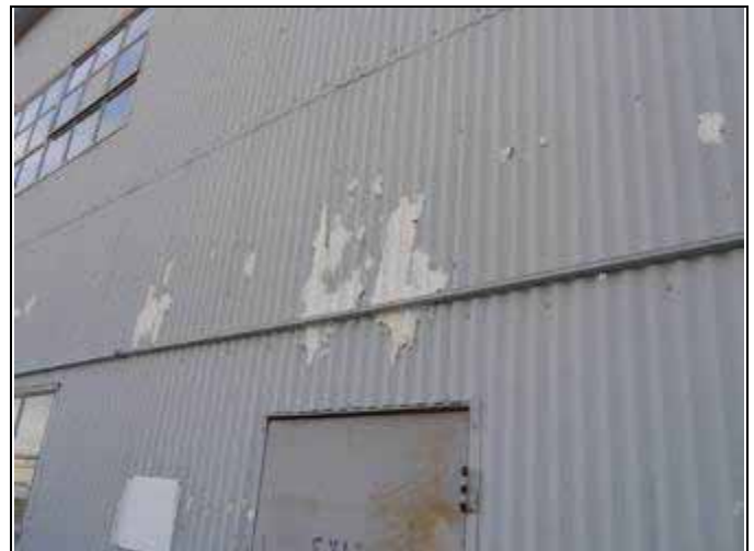
78. Peeling paint on wall panels
