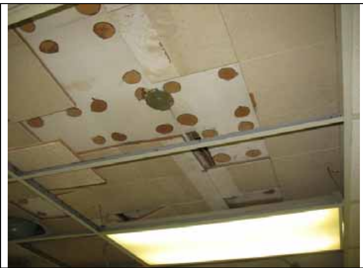
7. View of ACBM mastic on ceiling in NE office area of east hanger.
