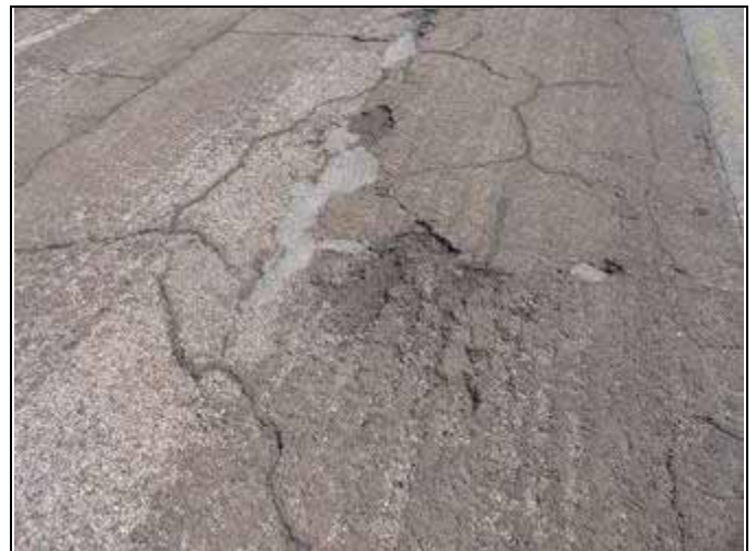
60. Pavement damage at south apron
