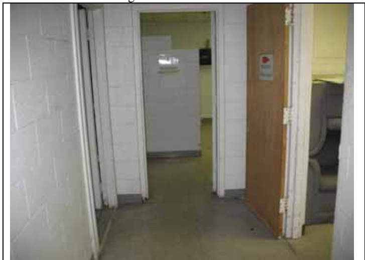
12. View of ACBM floor tile/mastic in 1 st floor room in NE Office area of east hanger
