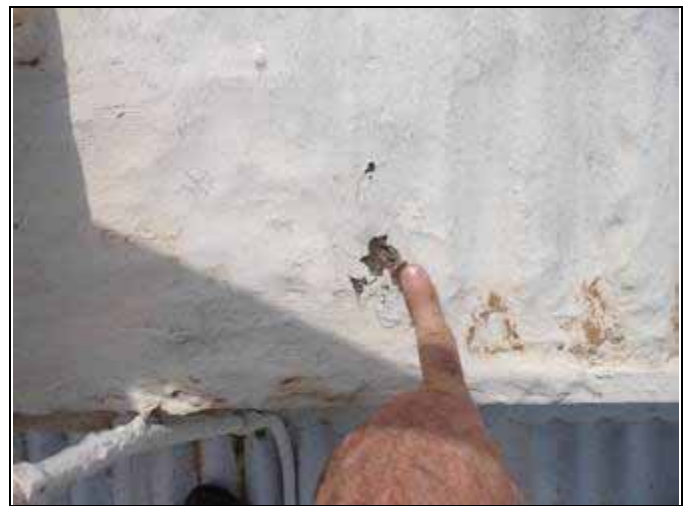
70. Deteriorate fabric of prior roofing repairs
