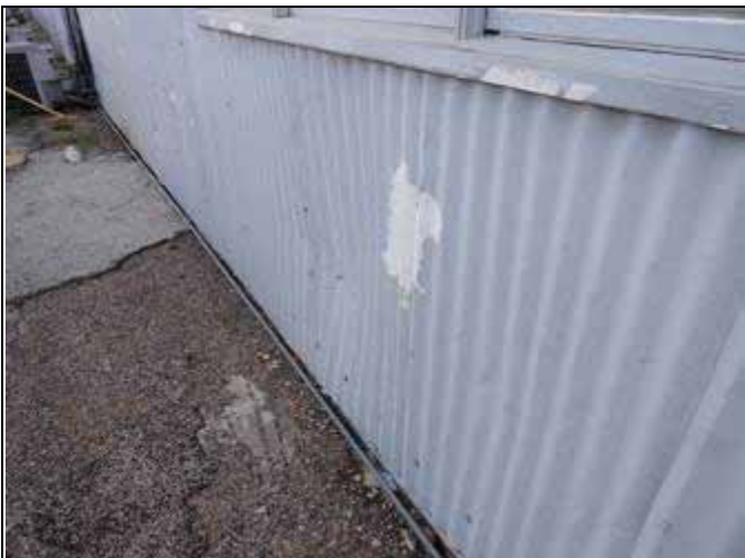
77. Impact damaged wall panels
