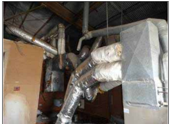
42. HVAC distribution ductwork
