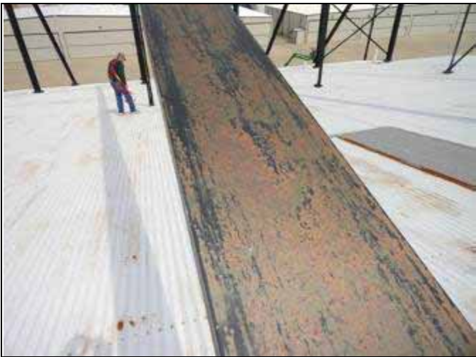
57. Surface corrosion at exposed roof structure
