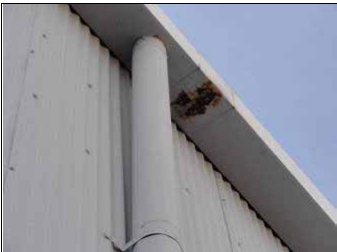
71. Corroded roof gutter
