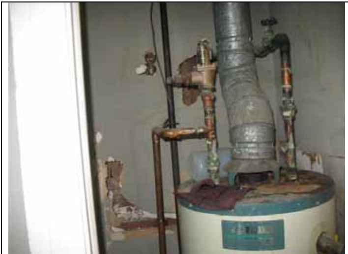
23. View of water heater in NE restroom of west hanger.
