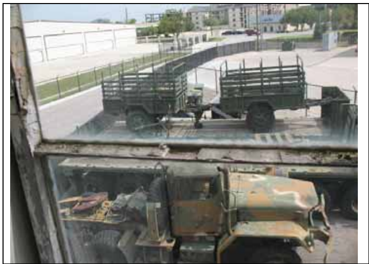
8. View of window pane on 2 nd floor above NE office area of east hanger.
