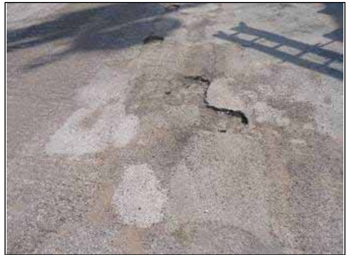
58. Paving damage at George Haddaway Drive
