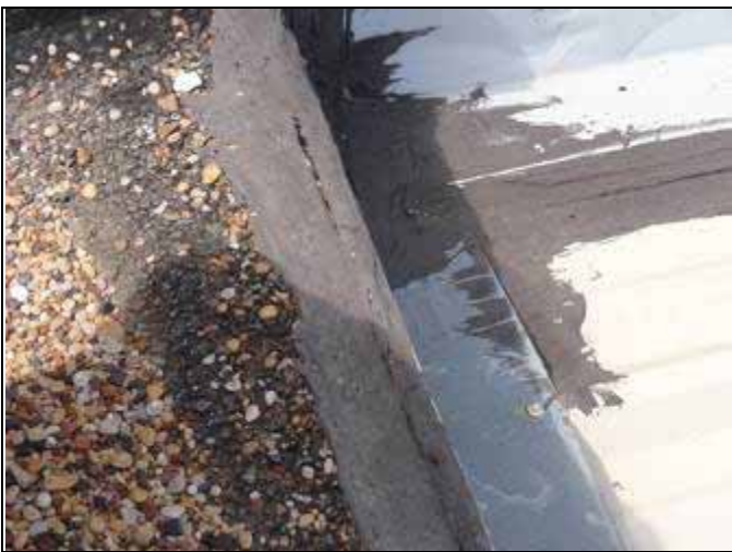
75. Split bitumen at built-up roofing
