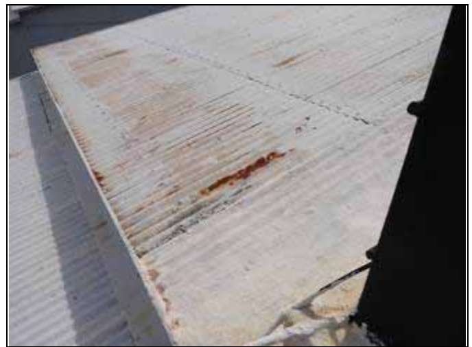
64. Roofing panel corrosion
