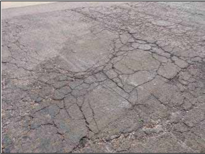
61. Pavement damage at south apron
