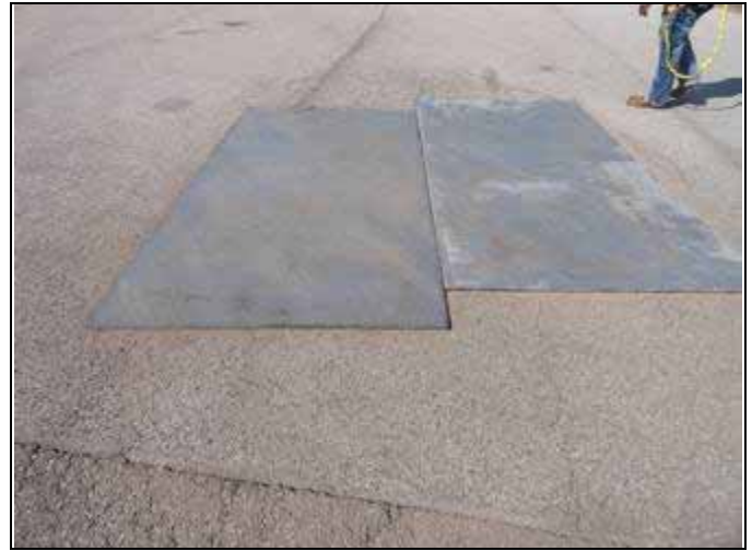
62. Steel plates set over pavement void at south apron
