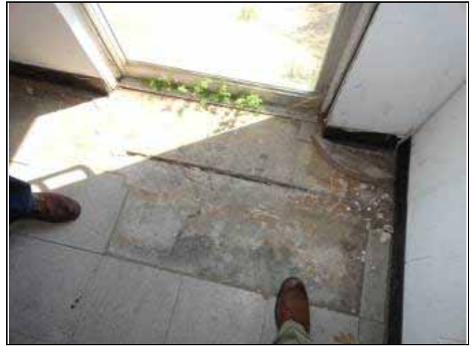
56. Minor slab displacement at east wall of 4730
