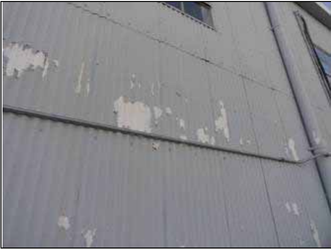
79. Peeling paint on wall panels
