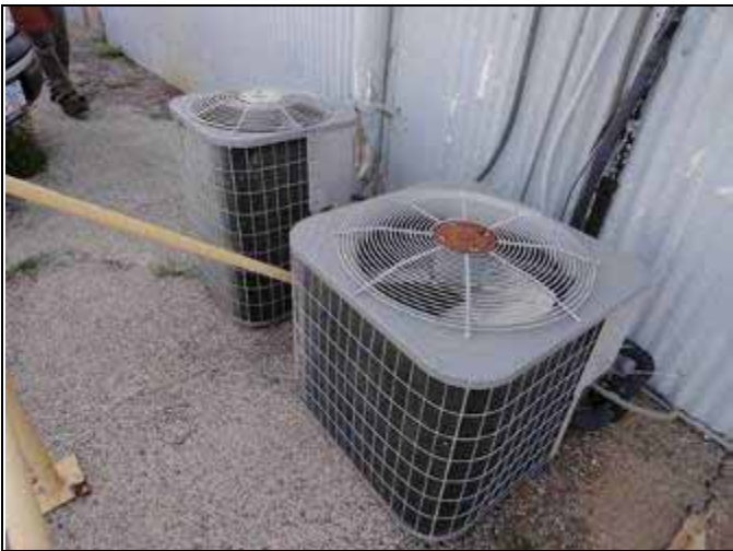
39. HVAC split system condenser
