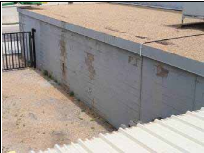
81. Peeling paint at addition
