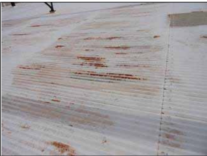
63. Roofing panel corrosion
