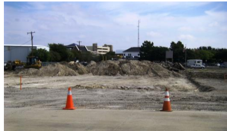
Above: piles of dirt at the Sky B&B hangar site.
