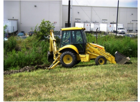
Above: Airport Maintenance clearing vegetation from a drainage channel on the west side of the airport.
