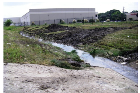
Above: the west side drainage channel is shown after vegetation and silt build-up has been removed. Keeping the channel clear is a perennial task that we eventually hope to render unnecessary by the addition of a concrete-lined channel with concrete side slope protection.
