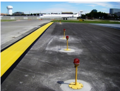
Below: runway end lights installed north of the EMAS bed. There is 35 feet of asphalt between the runway end and the beginning of the EMAS bed.
