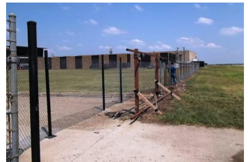
Below: Airport Maintenance Technician Tom Walsh erects temporary fencing to secure the airport perimeter until permanent repairs can be completed.
