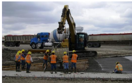
Below: a crew places concrete for the slope protection on the west side storm water detention area.
