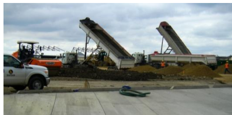
Above: trucks bringing in select fill to construct the base for the EMAS bed.
