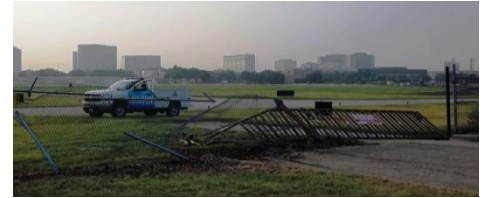
Above: Early one July morning, Airport Maintenance personnel arrived at the airport to find that the gate accessing the airport from Wiley Post Road – along with a section of the adjoining fence – had been hit and effectively destroyed by an unidentified vehicle.
