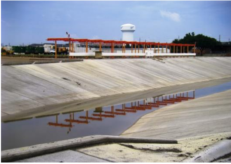
Above: concrete slope protection on the above-ground storm water detention area is nearly complete.
