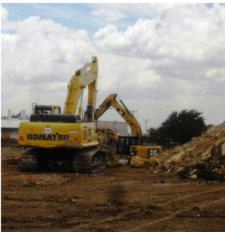
Above: excavators working in the Runway Safety Area as Phase 2 of the EMAS project gets under way.
