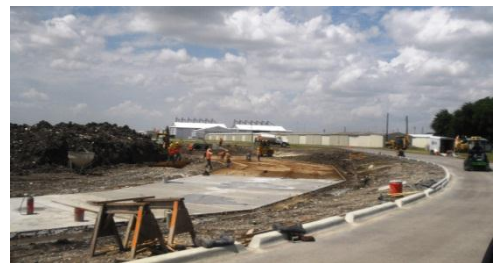
Above: the purpose of the concrete curbs is to keep vehicles from driving into the concrete-lined storm water detention areas. In this June 18 photo, the curbs have been placed and concrete is being placed on the bottom of the detention area. Additional concrete will be placed on the sloped sides.
