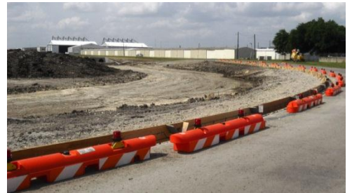
Below: grading work in progress on the east side of the detention area. Forms are set in place for concrete curbs along the south perimeter road (June 6).
