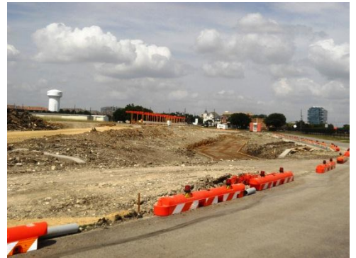
Above: fine grading is nearly complete for much of the above-ground storm water detention area south of the ILS localizer antenna; concrete forms are being set (June 6).
