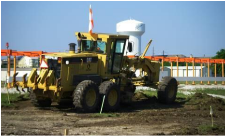
Above: a grader grubs grass and topsoil south of the Runway 15 Localizer antenna starting off Phase 1 construction activity for the EMAS installation.
