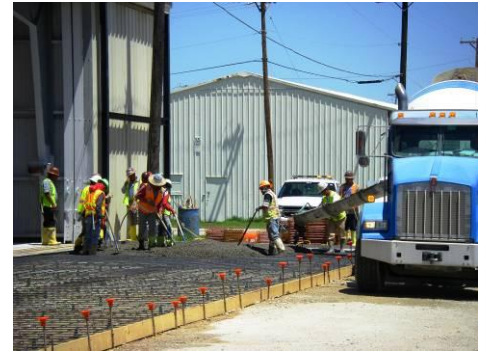
Above: The first concrete is poured on the S3 hangar ramp, part of the S1 & S3 ramp reconstruction project.
