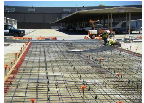
Below: forms and steel for the second concrete lane to be poured on the S3 hangar ramp. Note that this section includes a new drop inlet for improved drainage.
