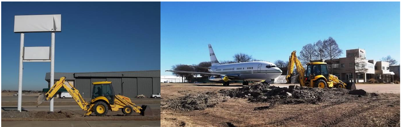
In mid-January, Airport Maintenance removed a light pole and a sign from the north side of the Jetport ramp. These fixtures were located in the object free area (OFA) on the south side of Taxilane Victor, creating a hazard for the larger aircraft (such as the Gulfstream G650) that have begun using Taxilane Victor in recent years.
