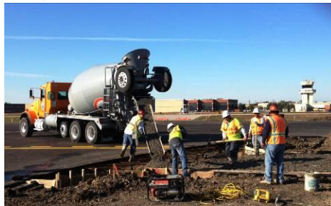
Above: pouring concrete to finish the east vehicle service road in the final construction stage for Taxiway Alpha.
