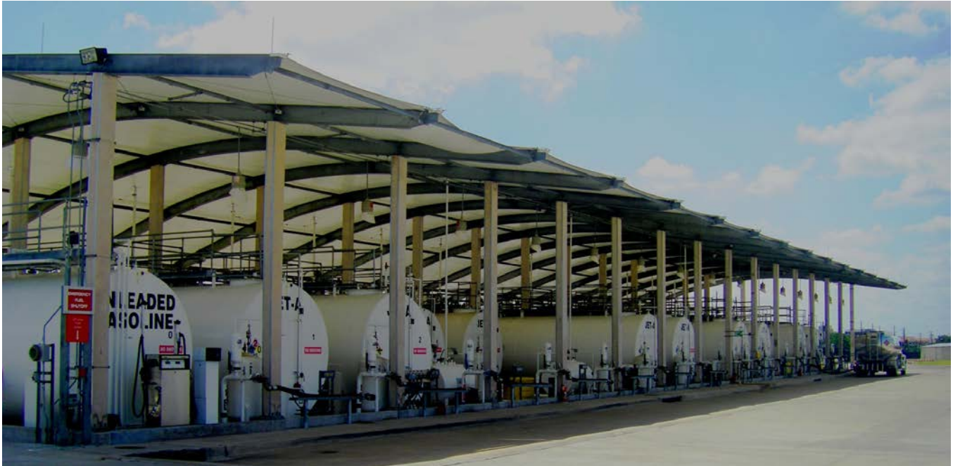
(Top) The Addison Airport bulk fuel storage facility (“fuel farm”). (Bottom) Conceptual Airport District boundaries.
