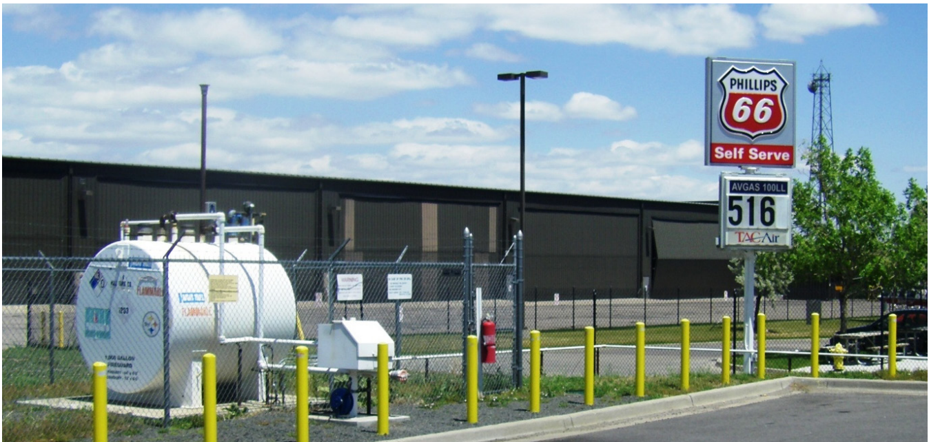
Self-service fueling facility at Denver Centennial Airport.
